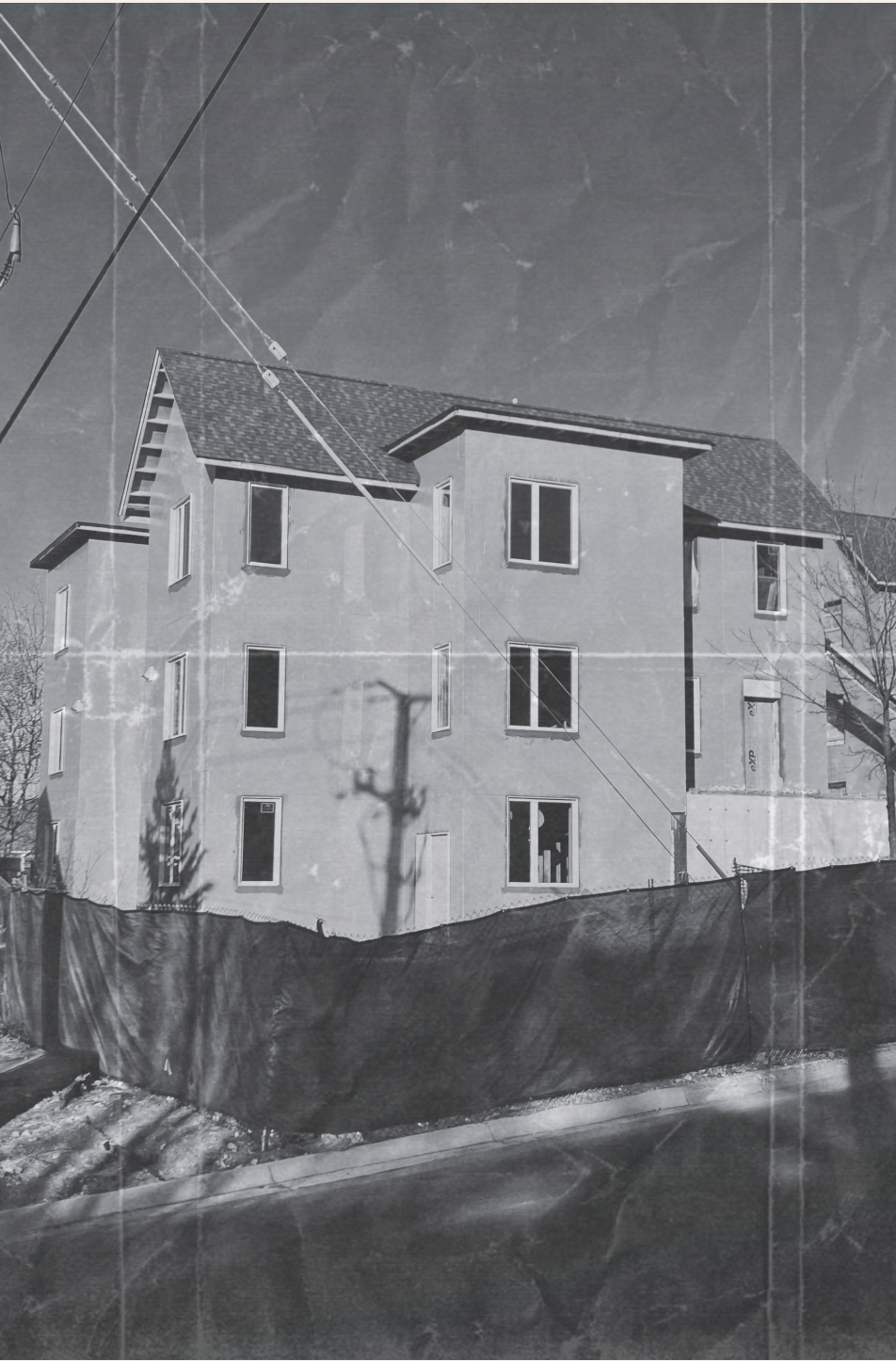
Our New Home Part 2: The protective walls of our home are built
